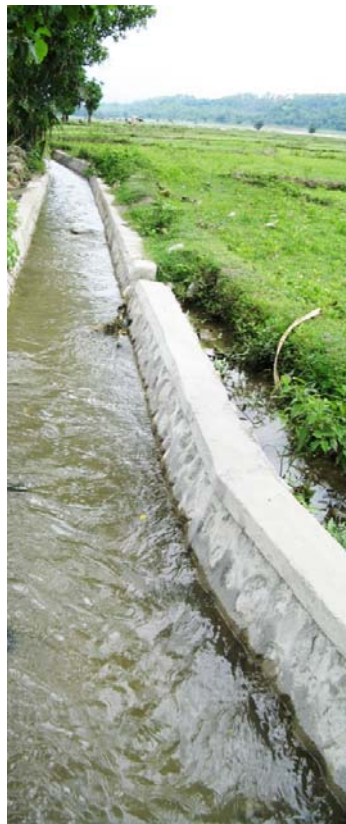
The rehabilitation of this irrigation system in the Marco Village, was funded by LDF allocated by the Cailaco Sub-District Assembly in Bobonaro District
